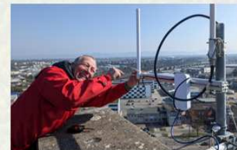
Installation LoRaWAN-GW HS Mannheim 2023
